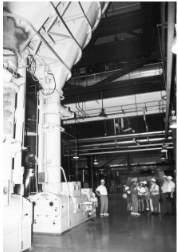
Members view the massive equipment at a Dairyland Power Cooperative generating facility on a previous tour.
